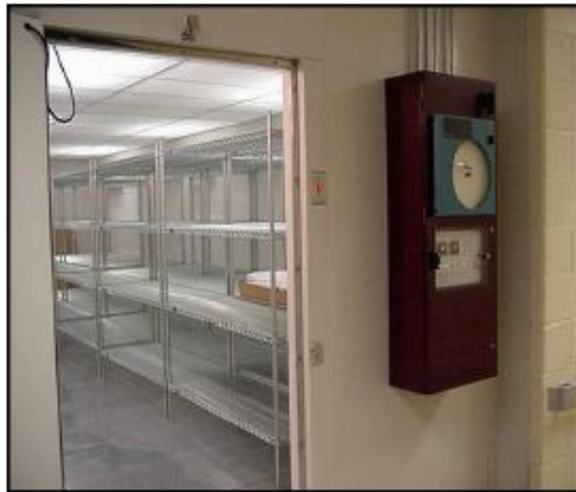
Pharmaceutical Laboratory Rooms
